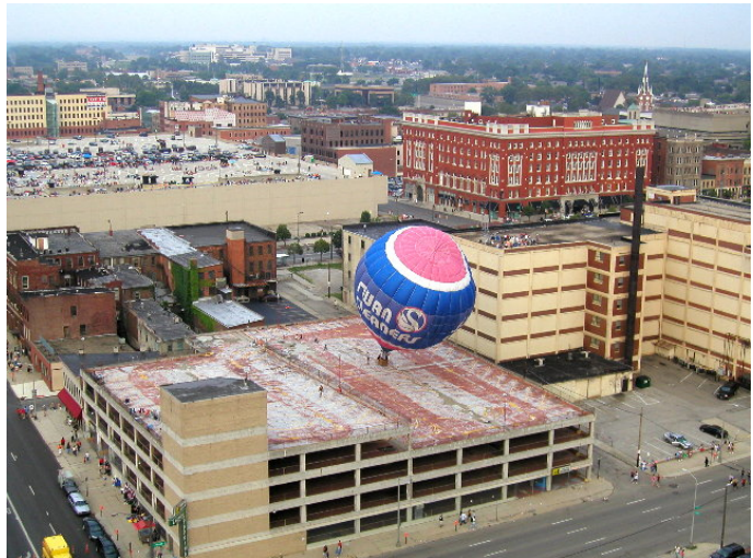
Here's a view of a parking garage roof just to our east. They were trying to launch a hot air balloon which never got off the ground because of excessive winds.
