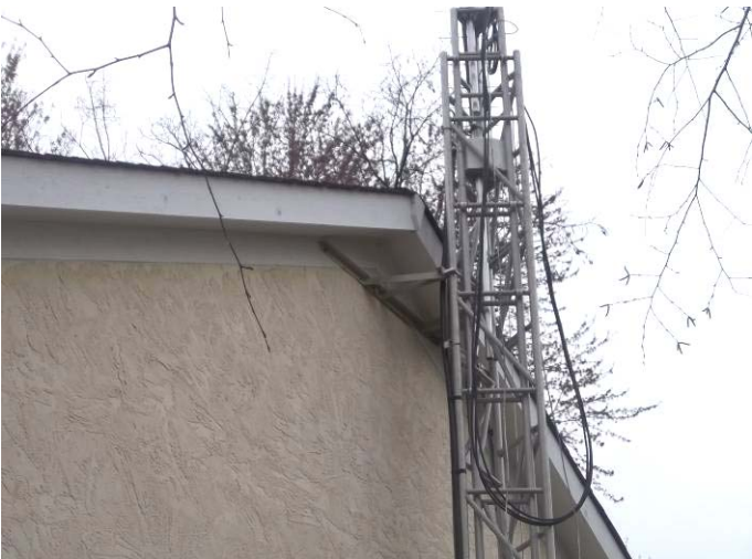
This shows the way I loop the coax lines that get extended when the tower is fully up. It's still early to tell if they will ever get caught on the tower end while extending or retracting. ...WA8RMC
