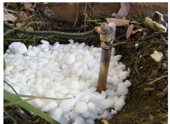
Figure III.4: The completed weld. Also seen in the pit are the water-softener salt pellets.
